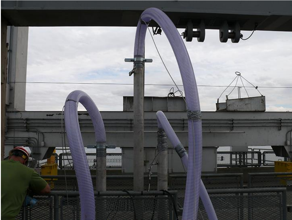
Figure 3.16. The STS lowered into the gatewell revealing the reinforced flex hose connected to the top of three SS injection pipes.
