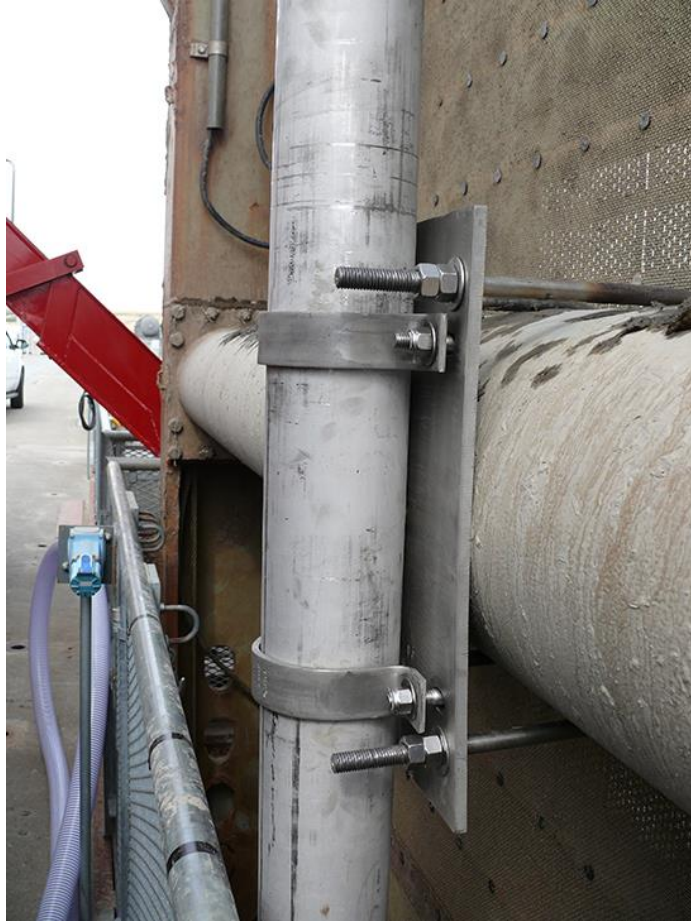
Figure 3.13. SF injection pipe top bracket plate is shown secured to the top STS frame horizontal pipe via SS U-bolt, pipe clamp, and hardware.
