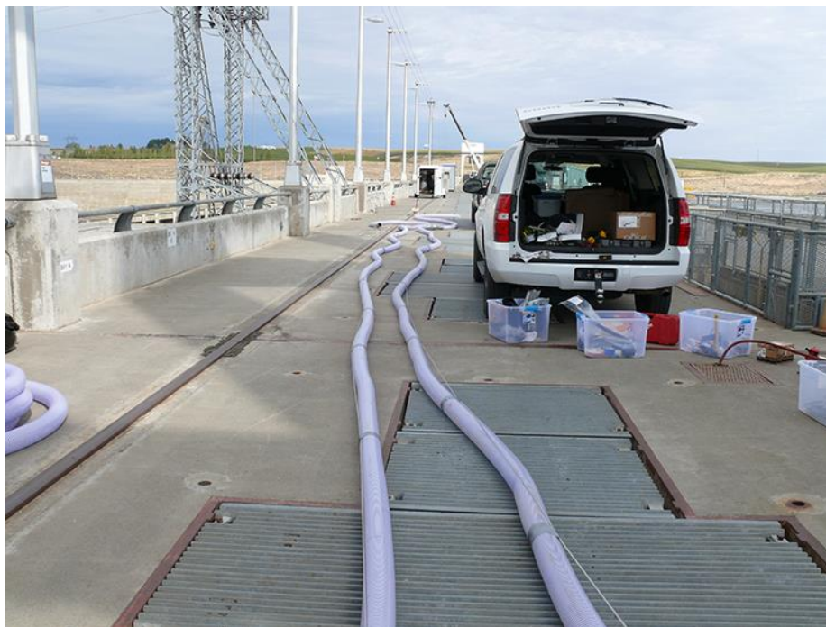
Figure 3.17. Four-inch-diameter flex hose is shown secured to .25-inch-diameter SS wire rope via hose clamps and duct tape.
